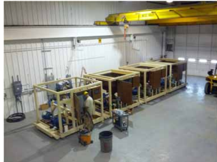
The slurry mix tank and 3 interconnected Ablation modules of the 5tph Unit
