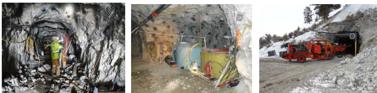
Figures 2: New Departure Silver Project: Mine Development at Laczay Adit and Tunnel
