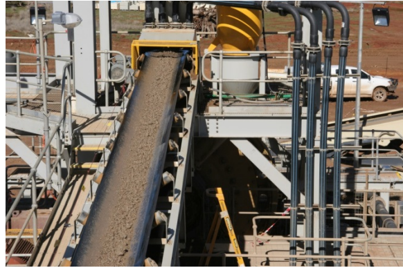
Oversize ore feed to ball mill
