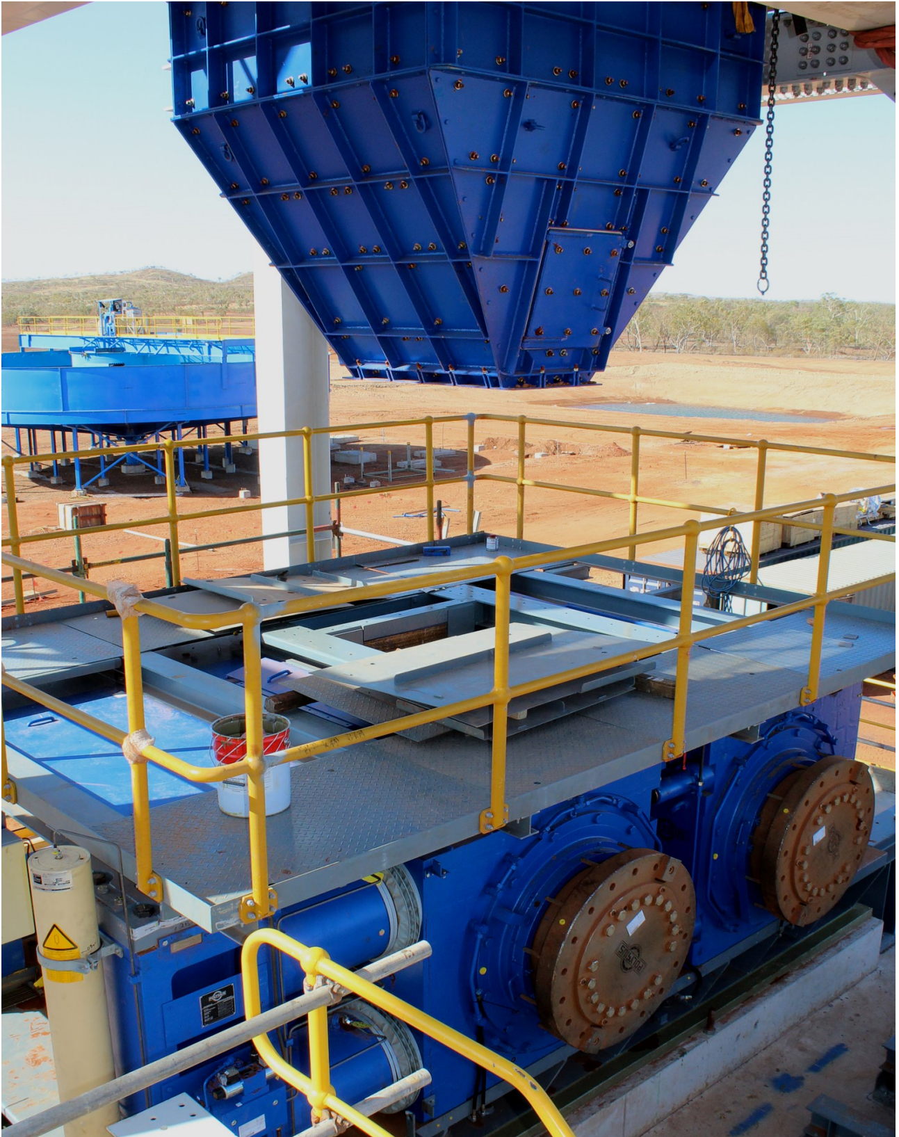
Figure 17: HPGR feed chute...see Figure 7 for location details
