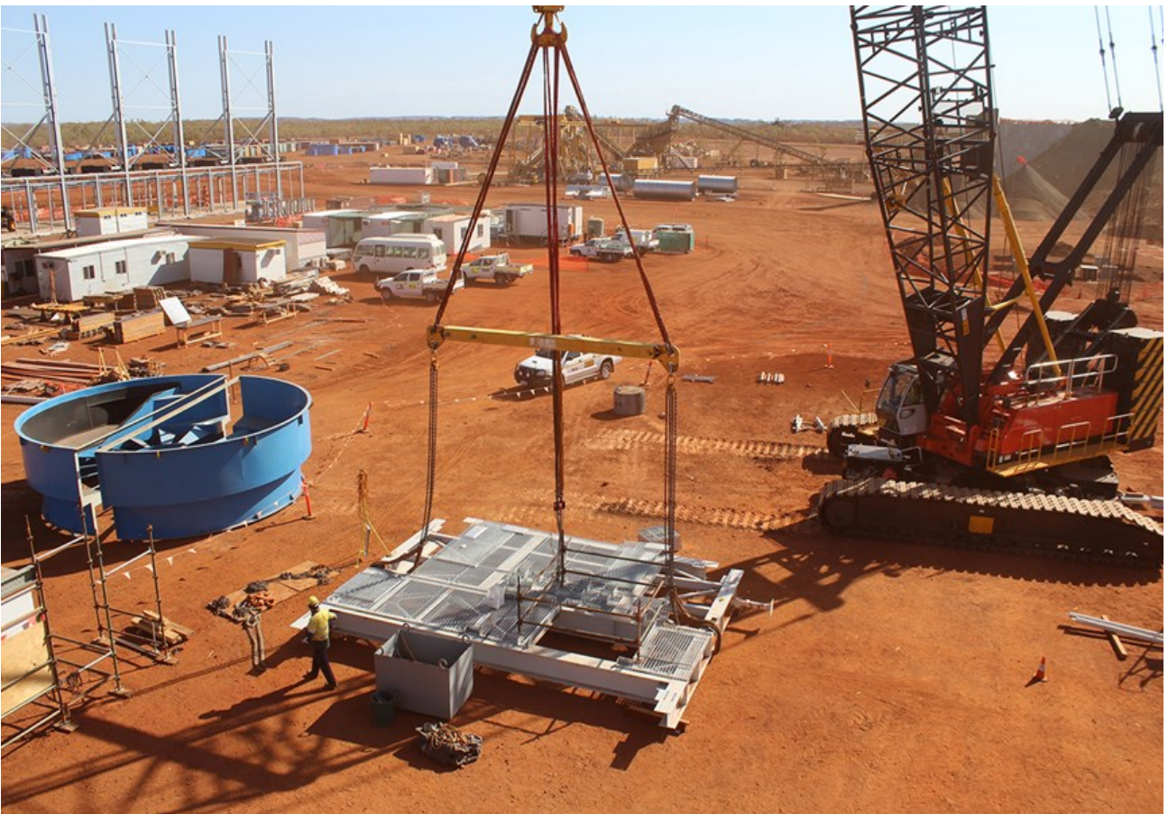
Figure 12: Upper platform for HPGR being prepared for lifting...see Figure 7 for location details
