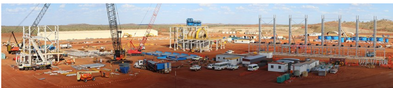
Figure 14: From left to right; HPGR, Ball Mill, Power Station and Flotation Cells in distant background...see Figure 7 for location details
