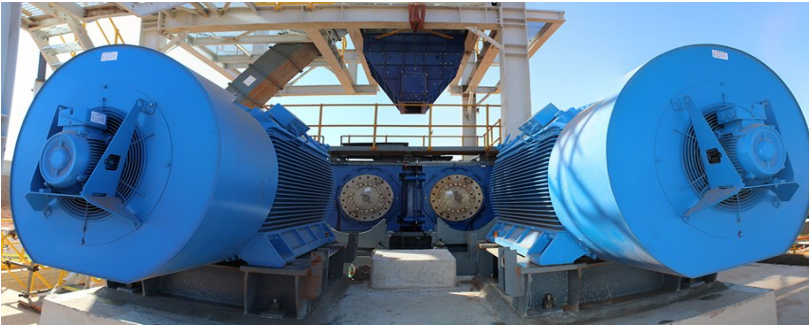
Figure 18: HPGR drive motors...see Figure 7 for location details
