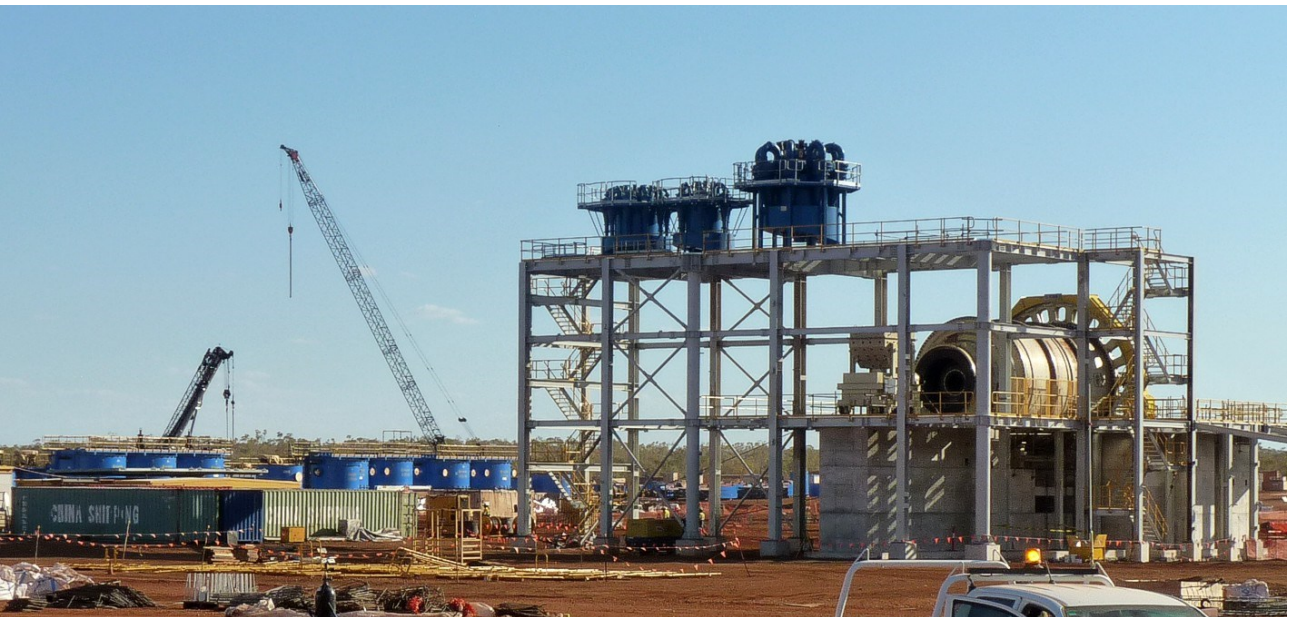
Figure 4: Ball Mill construction with Cyclones atop (right) and Flotation Cells in far background (left)...see Figure 7 for location details
