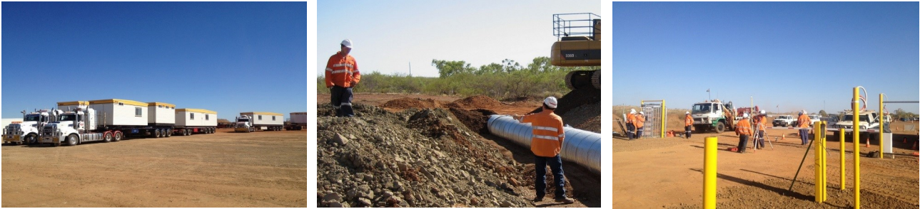
Figure 30: (From left to right); Site offices arrive at Rocklands, culvert construction and security gate entry upgrade...see Figure 7 for location details
