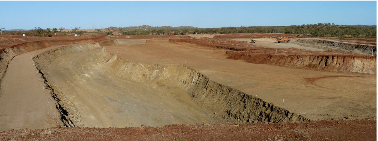
Figure 33: North-west end of LM Open-cut, with overburden and waste removed either side of the ore, which remains in-situ ready for future removal....see Figure 7 for location details
