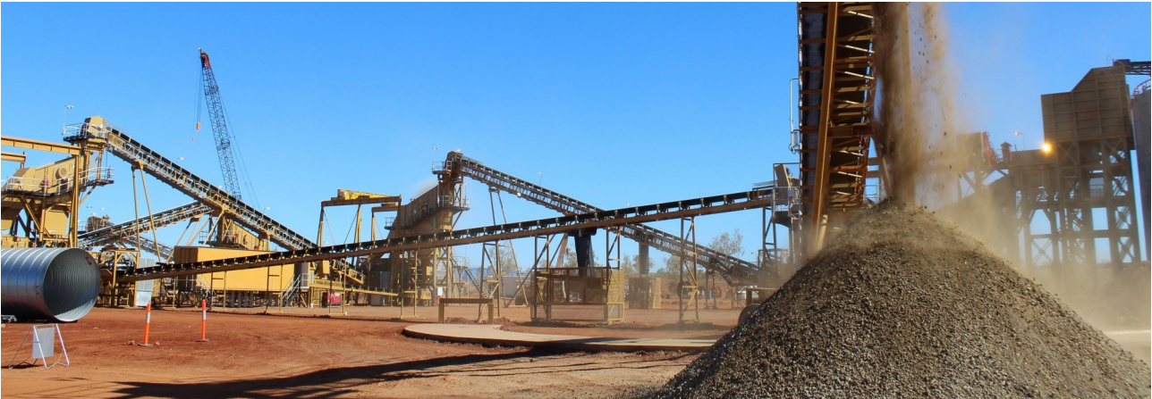
Figure 8: Crushing Circuit during recent commissioning ...see Figure 7 for location details
