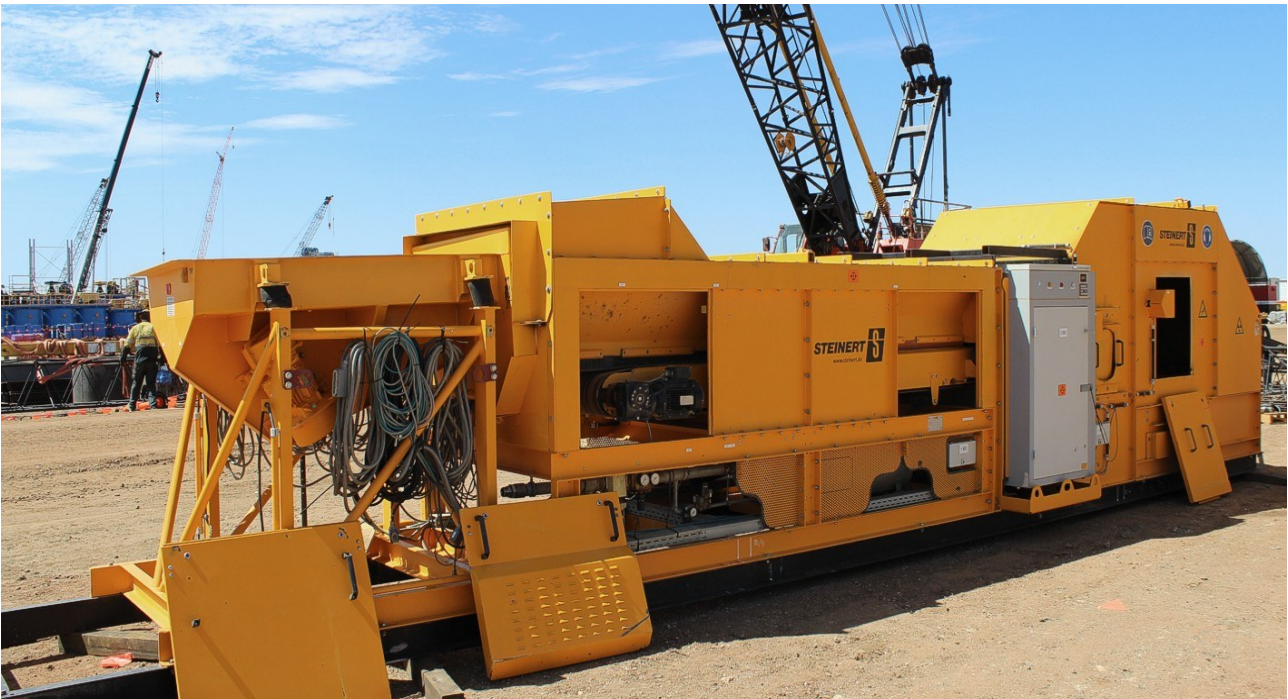
Figure 9: Ore-sorter being assembled at the Process Plant lay-down area, prior to being lifted into a temporary location at the Crushing Circuit where it will initially process native copper dominated ore types.
