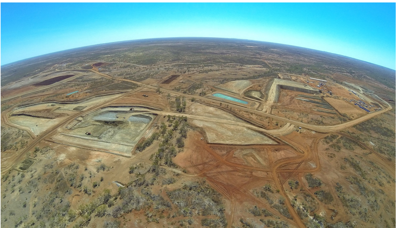
Figure 6: Aerial view of current work areas of the Rocklands Copper Project, including LM Stage-1 DSO Pit in foreground, water storage facility far left background, and ROM pad and plant site far right background.
