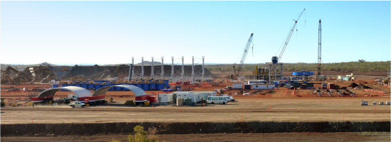
Figure 2: Process Plant construction from left to right; Crushing Circuit (far background), Flotation Cells (blue), Power Station (white steelwork), Ball Mill, Gravity thickener (blue) and Table foundations (right)...see Figure 7 for location details
