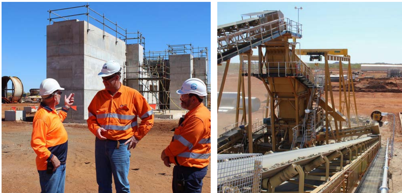
Figure 11: Left Image; Executive Chairman Peter Hutchison, Mine Manager (SSE) Andy Keogh & Process Manager Rob Brougham inspecting the Ball Mill Foundations. Right Image; Conveyor 7 of the crushing circuit during commissioning test crushing.
