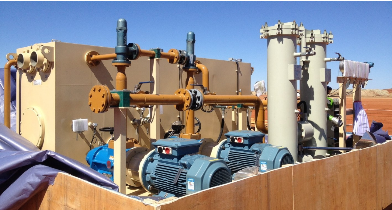
Figure 16: Delivery audit - lube system for Ball Mill main bearing and pinion
