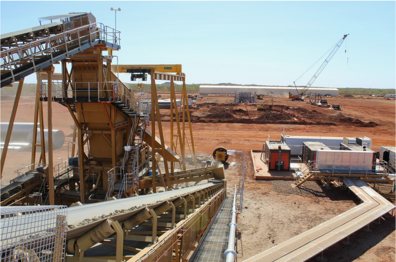
Figure 8: The crushing circuit undergoing commissioning (foreground), major earthworks commence at the site of the gravity circuit (middle distance), concrete foundations for the ball mill (background) and Process Plant Stores shed (far background). The site of the HPGR is obscured by the crushing circuit (middle distance to the left of the image).
