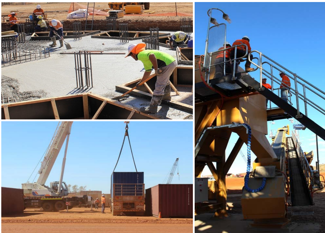
Figure 12: Clockwise from middle left; Concrete pour at the Tailings Thickener; commissioning meeting at the crushing circuit and; unloading component deliveries at Rocklands.
