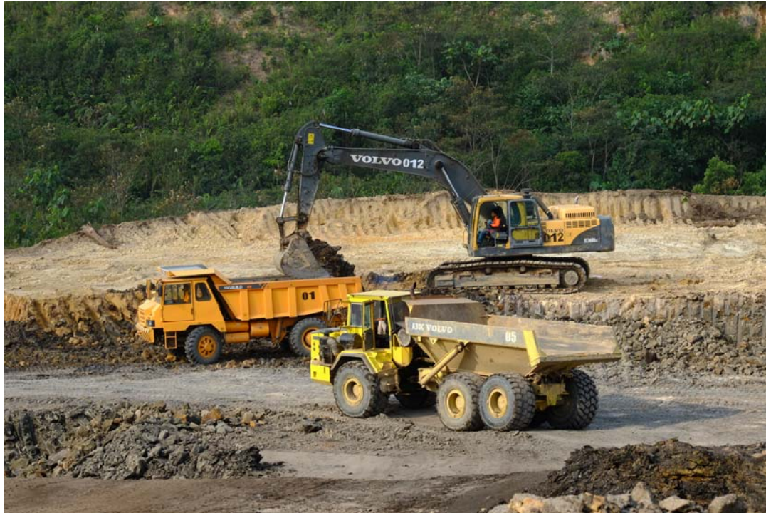
Figure 2: Overburden stripping commenced at a new location in Block 1 of Pit 2 in accordance with the designed mine plan
