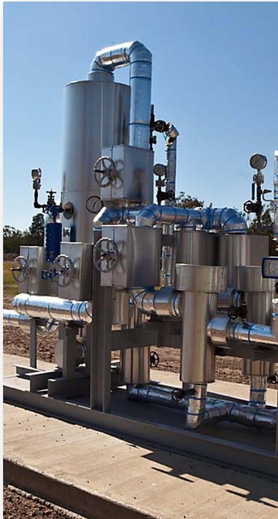
Liquid Knock Out Module Bloodwood Creek Queensland
