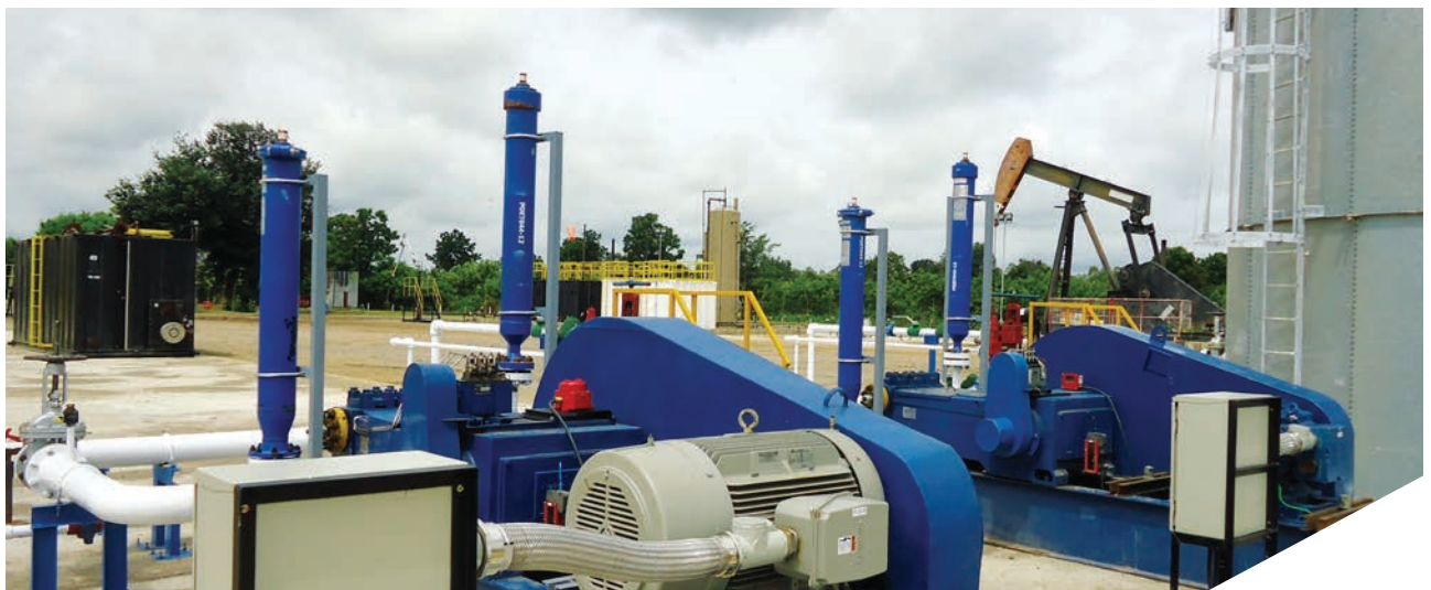
Figure 3: Water flood injection equipment on-site at WBEXT-1 well site
