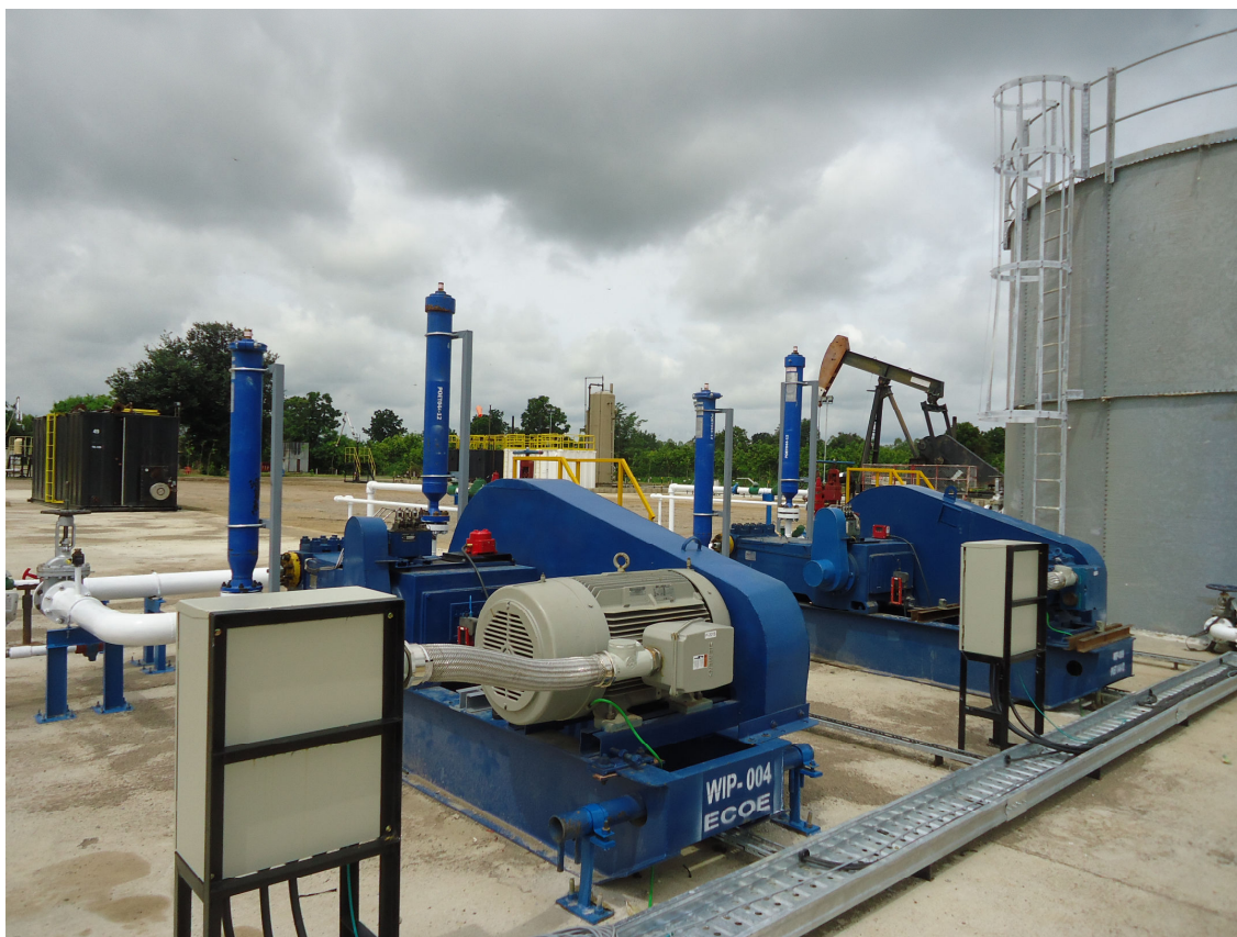
Figure 3: Water flood injection equipment on-site at WBEXT-1 well site
