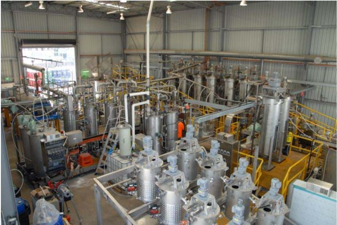
Stage 1 Test Plant with Stage 2 module in the foreground
