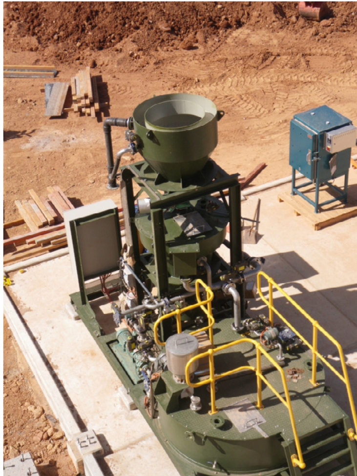
Figure 6. Acacia reactor in position.
