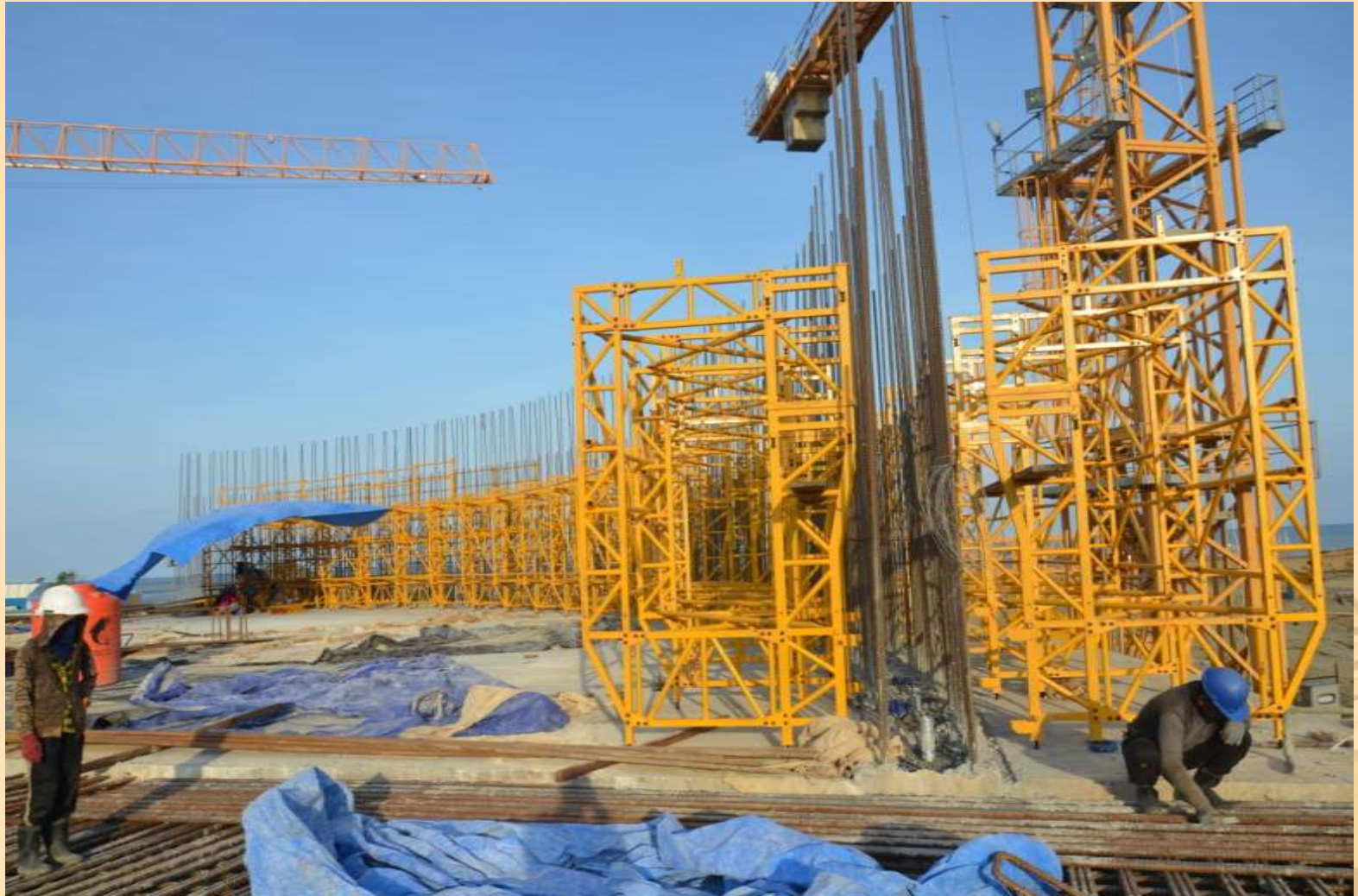
Casting of Base Slab Segments 5 & 6 completed with installation of Slipform Equipment in progress
