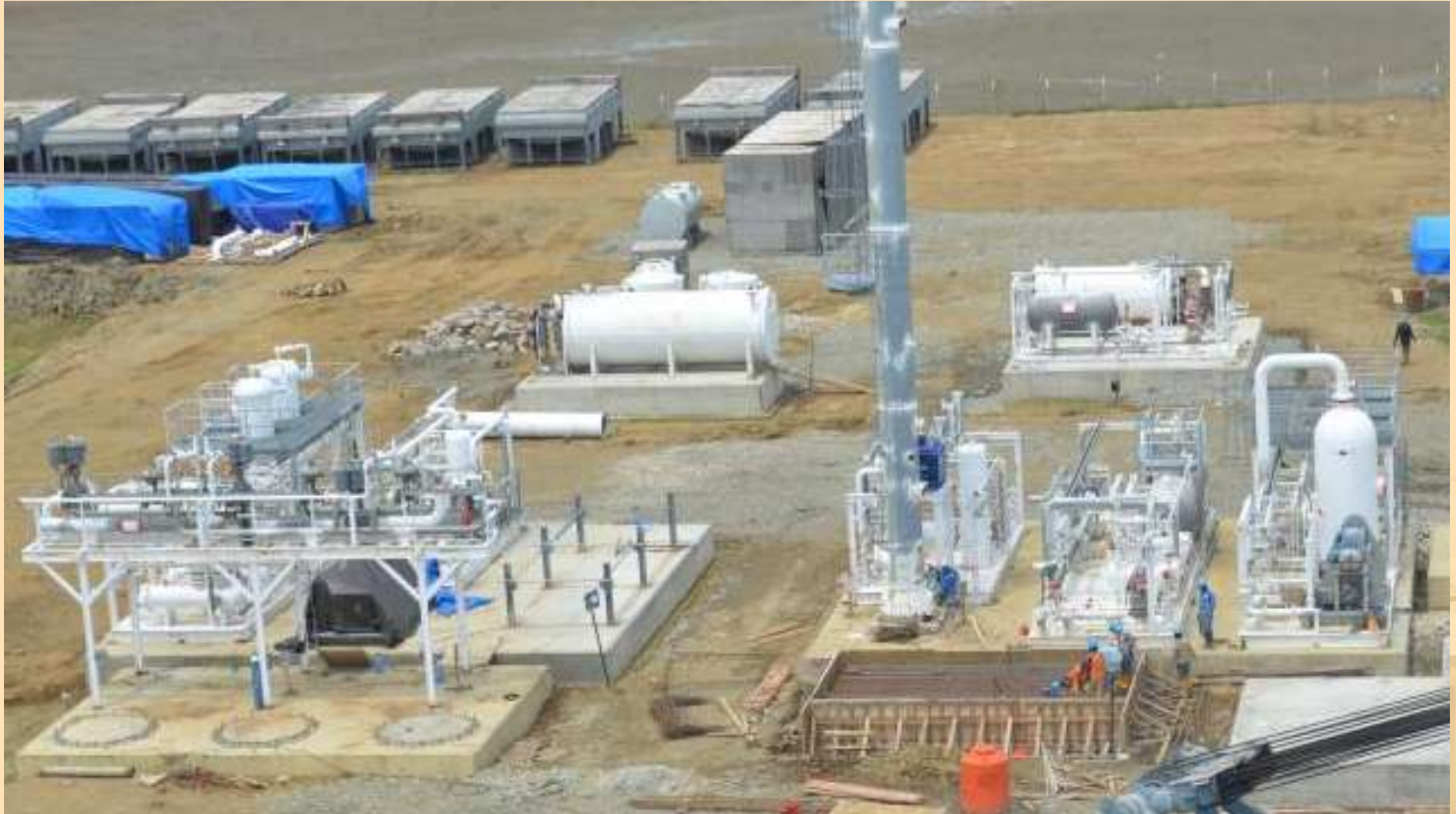
Main Processing Plant Area - Train 1 of Pre-treatment Plant
