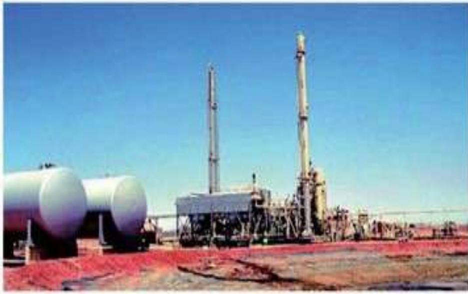
Eromanga Gas Plant, Australia
