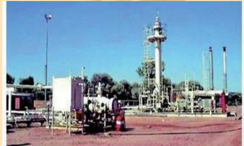
Gilmore gas plant, Australia
