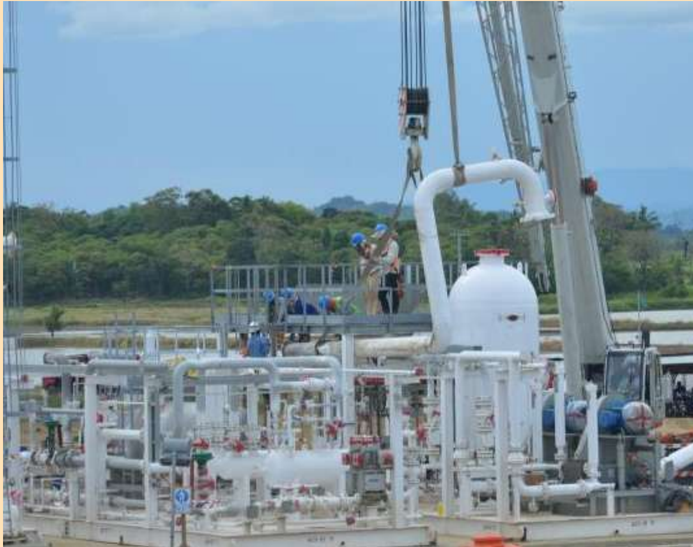
Main Processing Plant Area - Train 1 of Pre- treatment Plant
