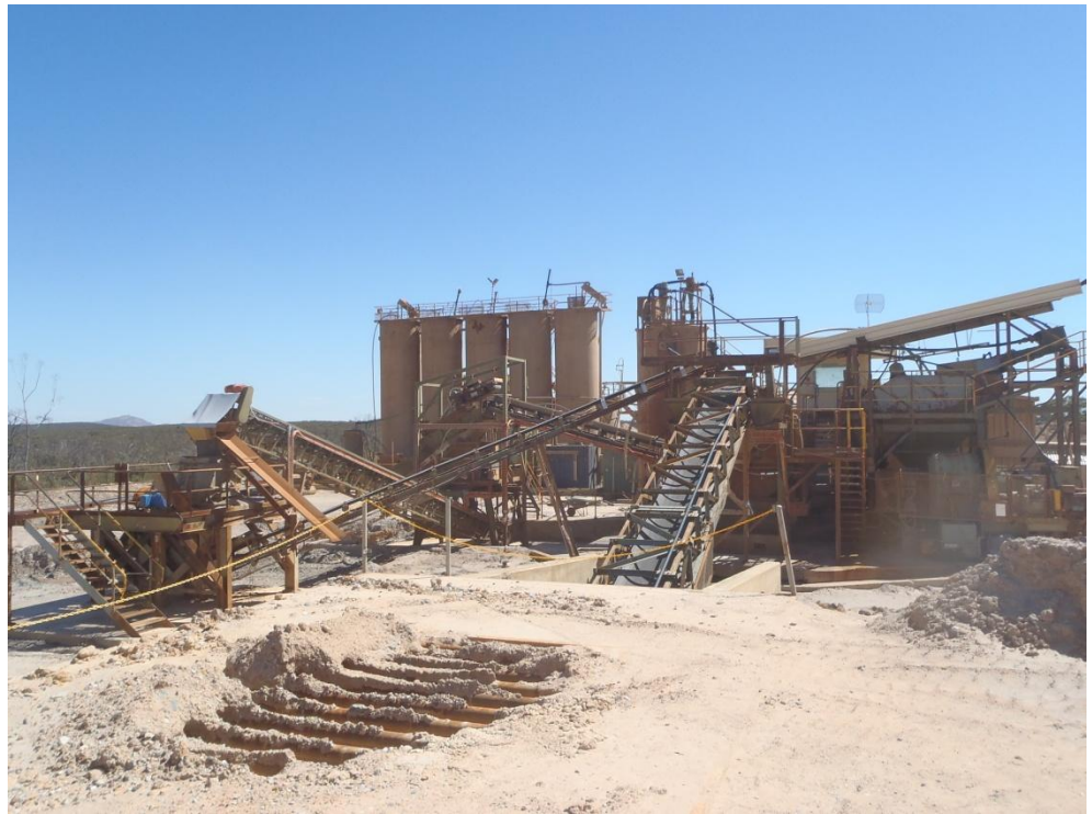
Maxwell Mill – crushing and gravity circuit viewed from in ground feed bin
