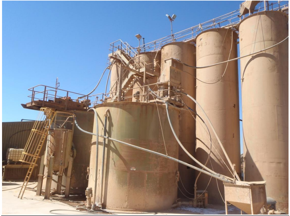
Maxwell Mill – CIP circuit - Agitator and Pachuka tanks
