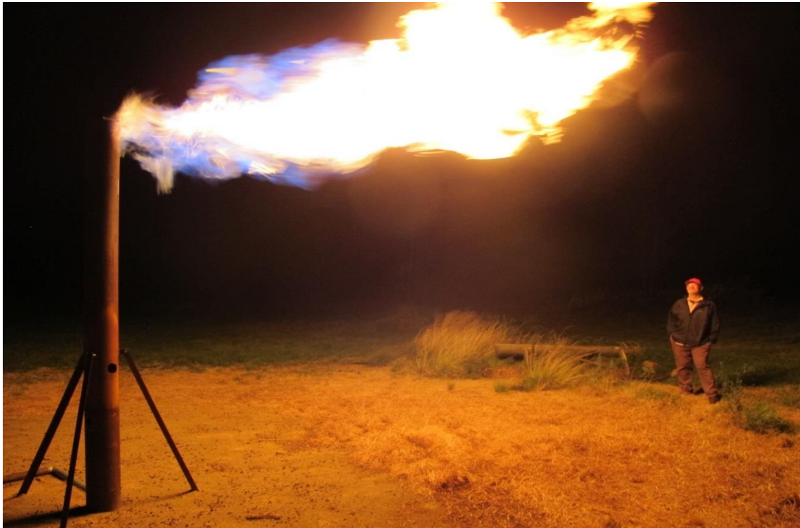
Photograph of Hole KA-03PTR flaring gas
