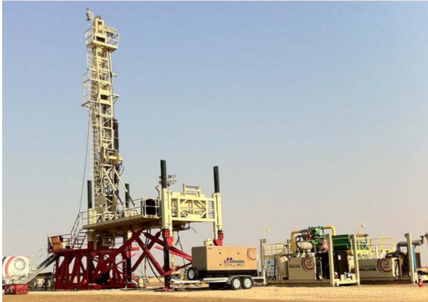
Example of drilling rig set up to core – max depth to 2500m
