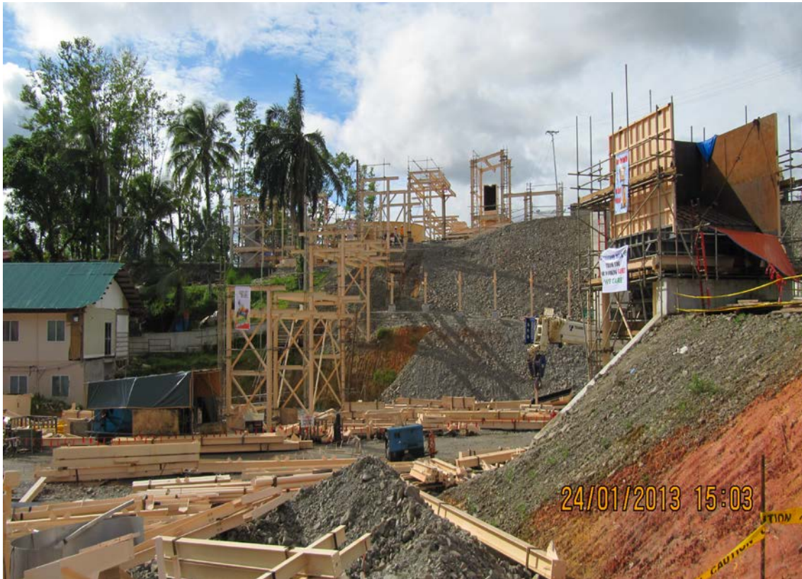
Photo 3. Pipe rack construction from SAG mill to leaching circuit on the left with the emergency feed station on the right.
