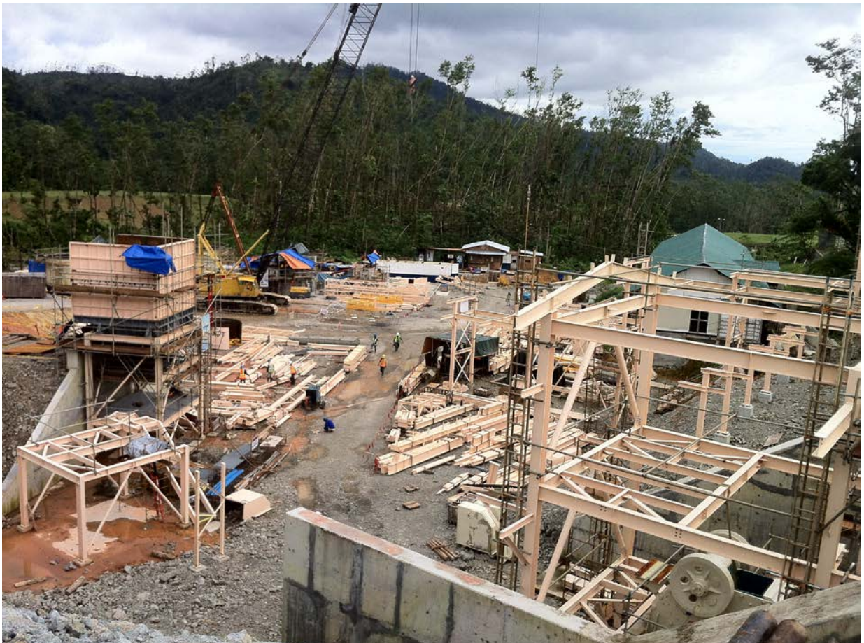
Photo 2. Installed crusher on the right and emergency feed station on the left. The SAG mill foundations are behind the 150 tonne crane which will be used to lift the SAG mill components onto the concrete foundations.
