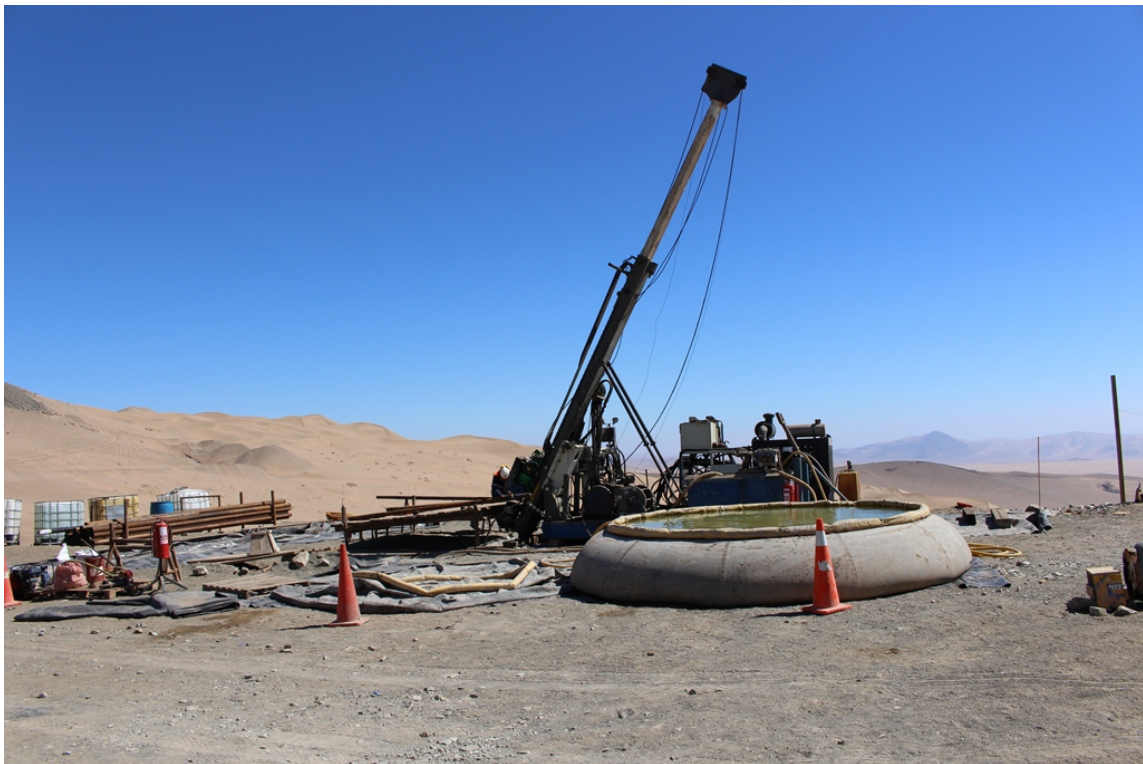
Figure 2 – Drill rig setting up at the site of the first ever diamond drill hole drilled at El Roble targeting beneath current mine at Descubridora vein.
