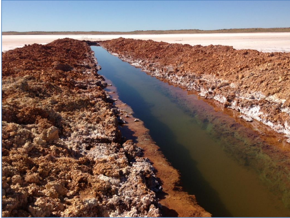
Curtin Boundary Trench 2m deep dug into fractured siltstone prior to pumping.
