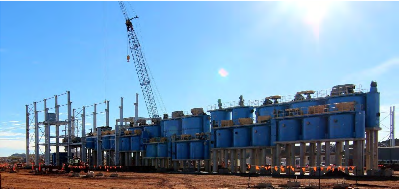
Figure 24: Flotation circuit building under construction showing smaller concentrate collector tanks in the foreground
