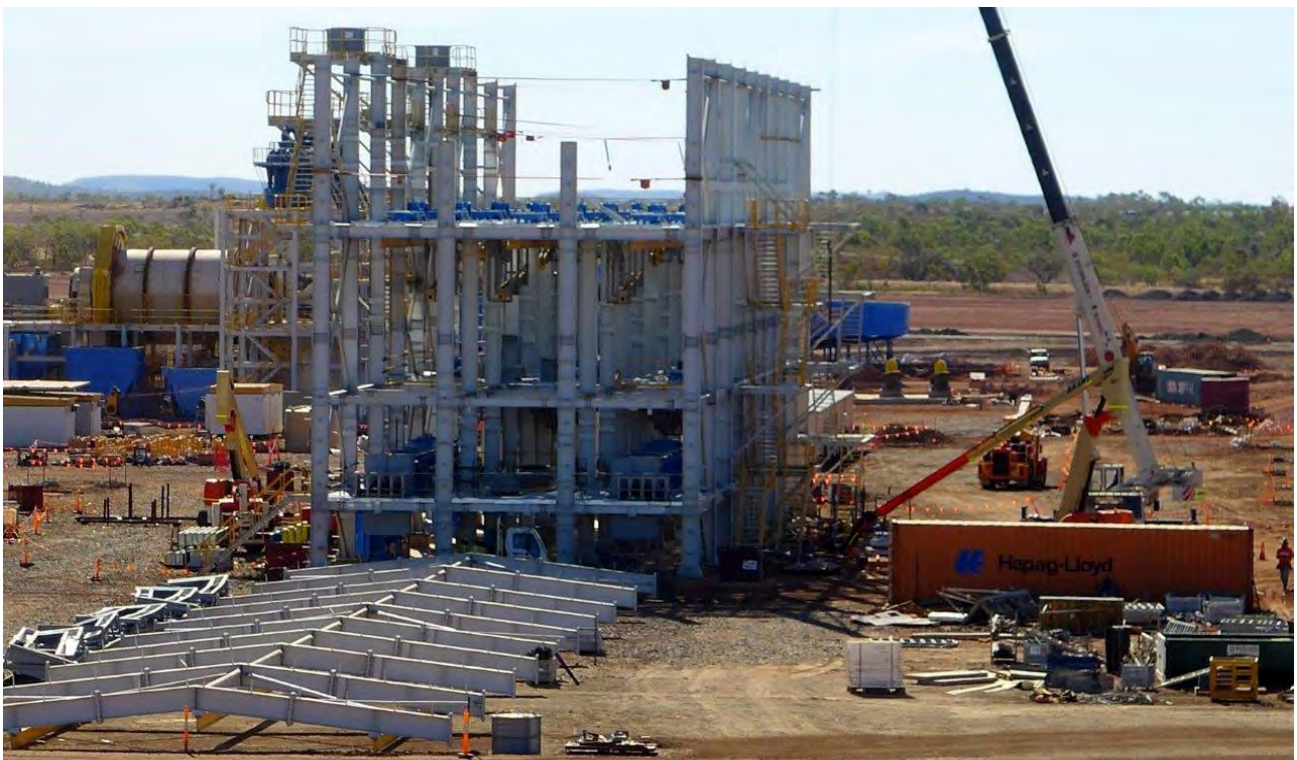
Figure 27: Tables Separator Building, with pre-assembled roof structure in the foreground prior to lifting into place
