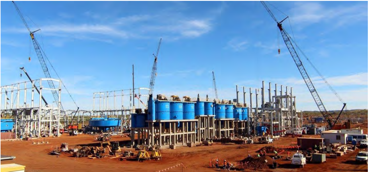
Figure 22: Flotation tanks, Cu circuit on the left and Co/pyrite circuit on the right, and Cu and Magnetite regrind Tower Mills in the background
