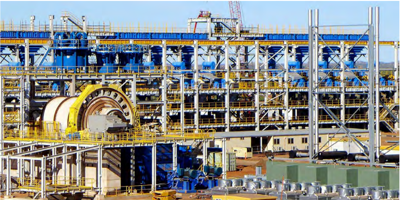
Figure 16: Ball Mill in foreground, gravity jig building in background
