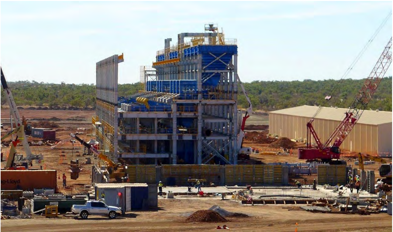
Figure 26: Gravity Jig Building, now dwarfing the Company's warehousing complex (right); Coarse Native Copper Concentrate Storage shed formwork in place for next concrete pour.
