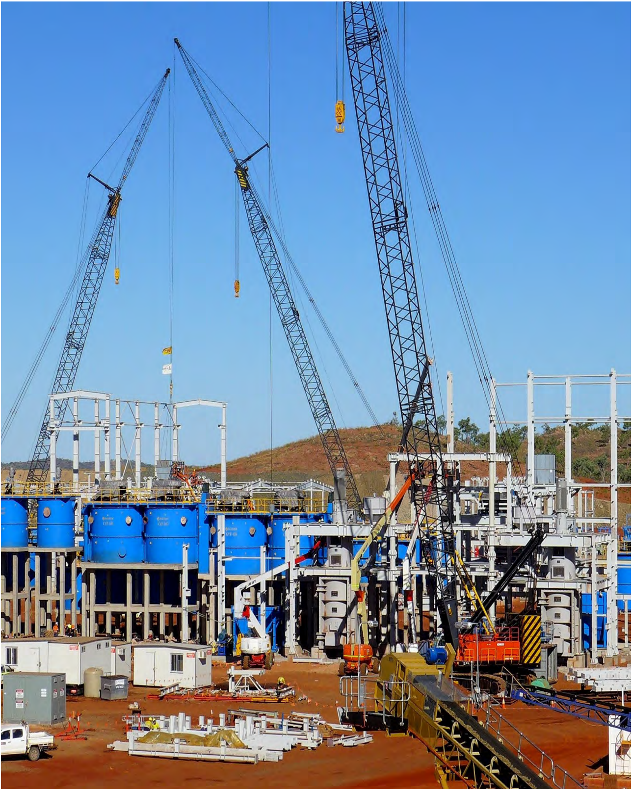
Figure 4: Steel erection at the flotation Cells (left) and Cu Regrind Mill (centre) in the Flotation circuit. Magnetic separation and Regrind Mill (right)
