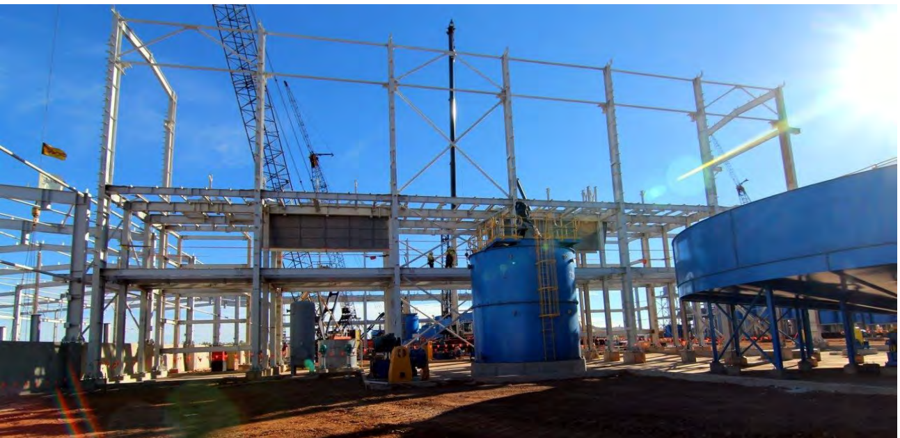
Figure 28 (top to bottom): Tables building (left) and Gravity Building (right); Ball Mill, Gravity Circuit and Power Station (middle) and; Copper Concentrate Filter Building under construction (Copper Concentrate Thickener to the right).
