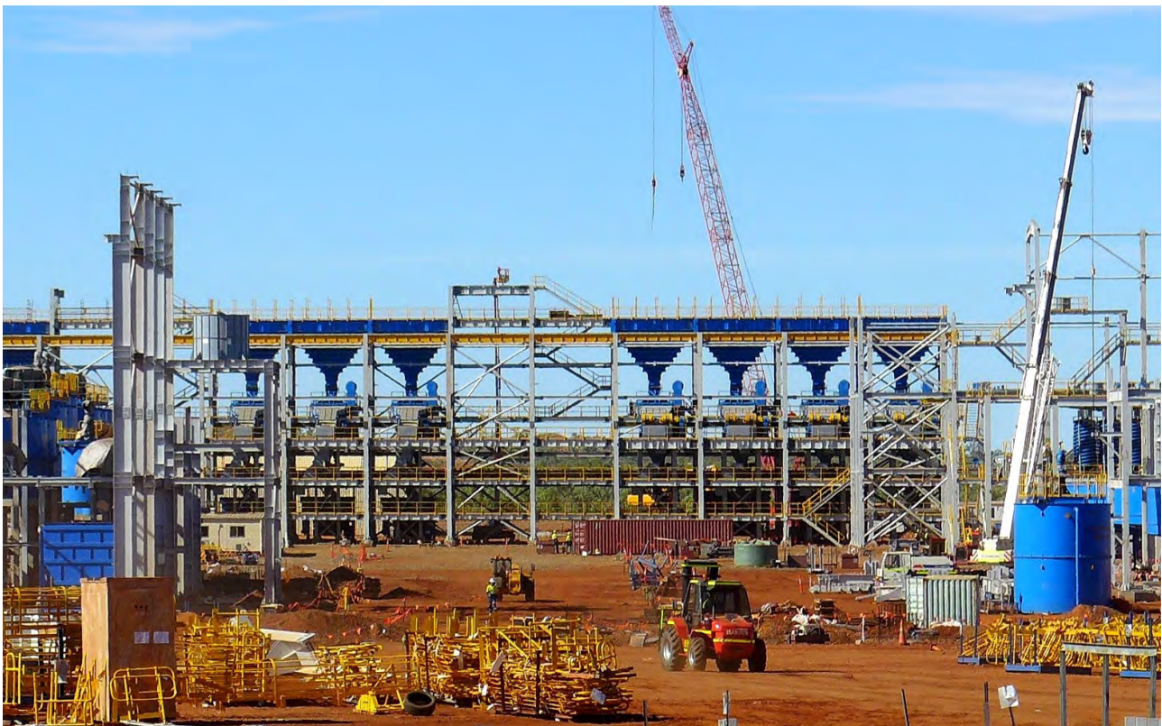
Figure 15: Jig Building showing the top floor (Jig Feed Distributor Conveyors)
