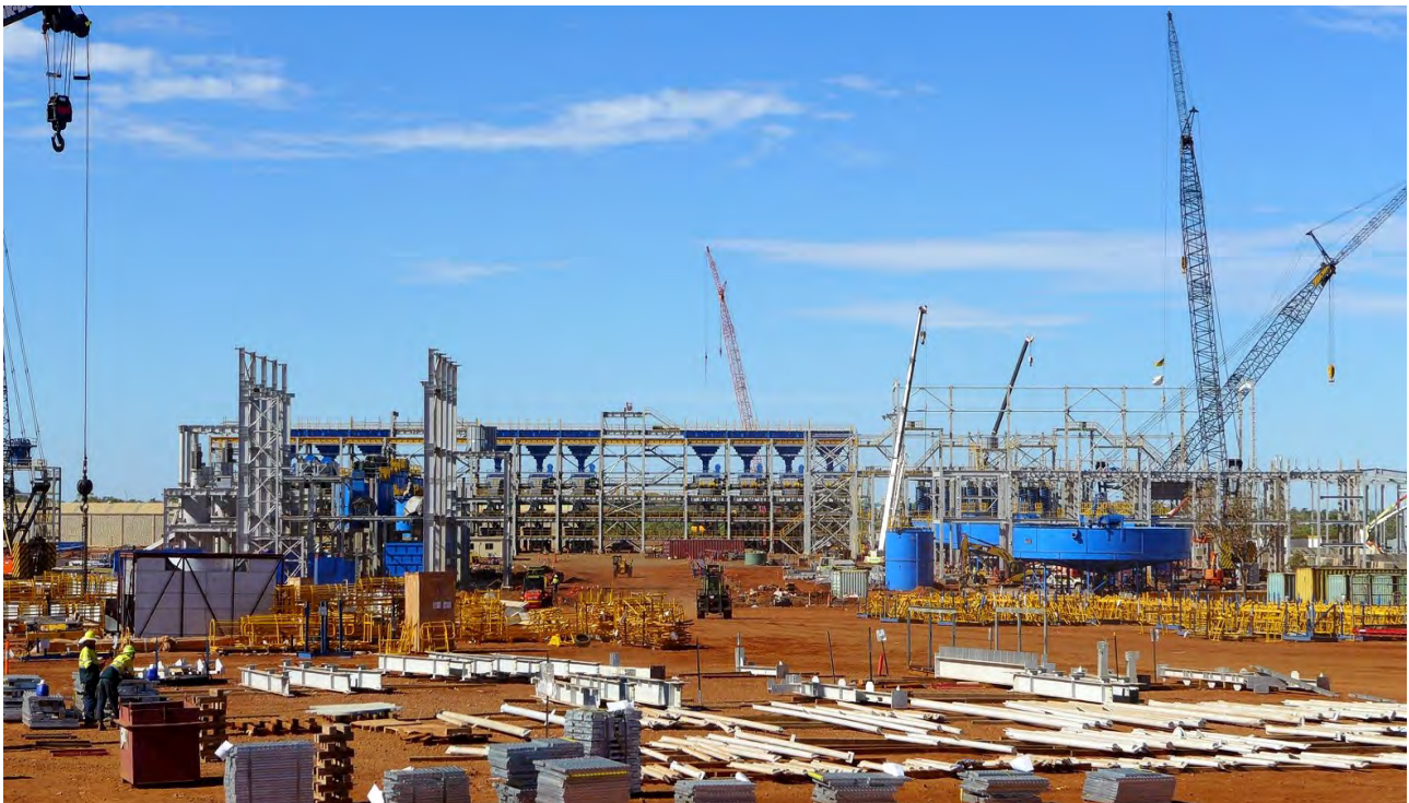
Figure 5: Rocklands Process Plant currently under construction (background) and lay-down and assembly area (foreground).
