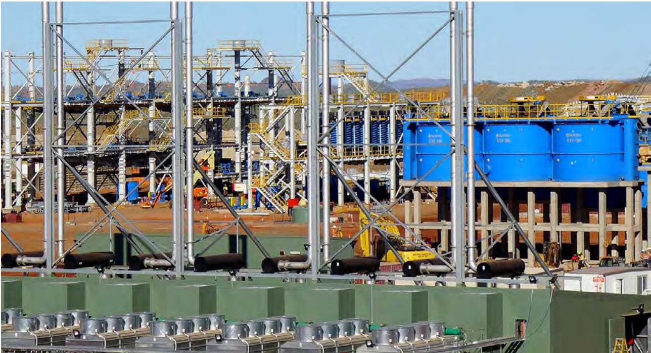
Figure 34: Power Station (foreground), Flotation Circuit (middle right), Spirals (centre background) and Gravity Jig Building (far left background)
