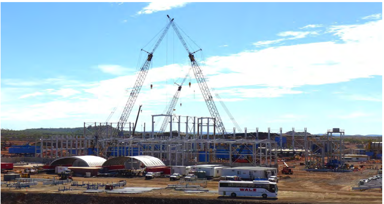
Figure 19: Temporary workshop area (domed structure) and concentrate storage buildings being constructed immediately behind.
