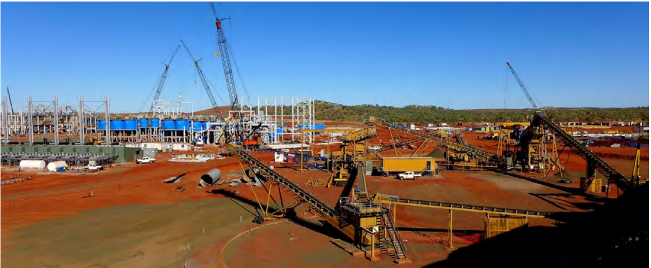
Figure 18: View from the ROM pad - Crashing Circuit (foreground) and from left to right; Power Station; Flotation Circuit and Cu Re-grind and Magnetite Re-grind circuits. Steel component deliver & lay-down area in background (far-right).
