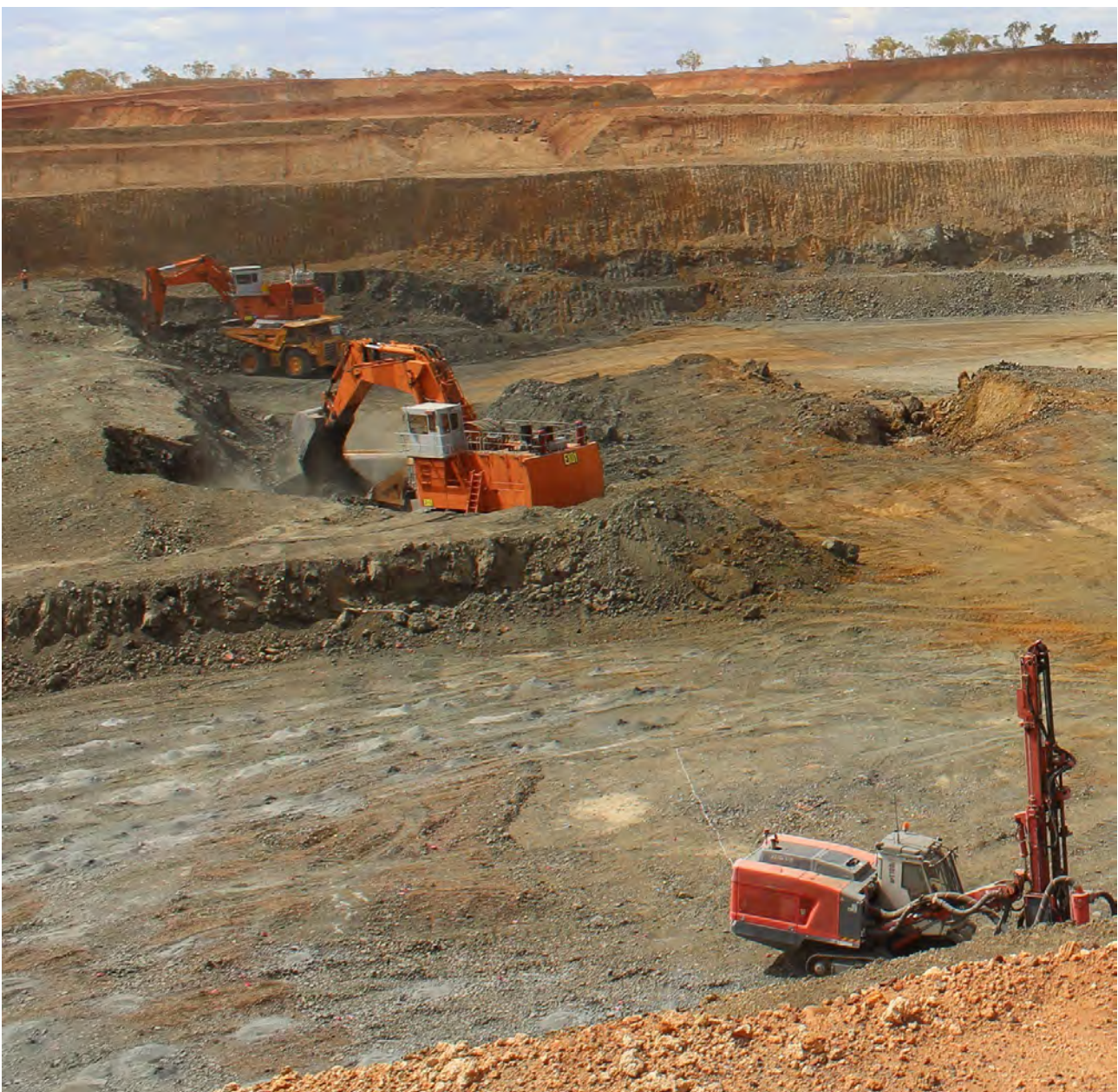
Figure 6: Two diggers in ore in LM1 Pit whilst blast-hole drilling continues in the foreground
