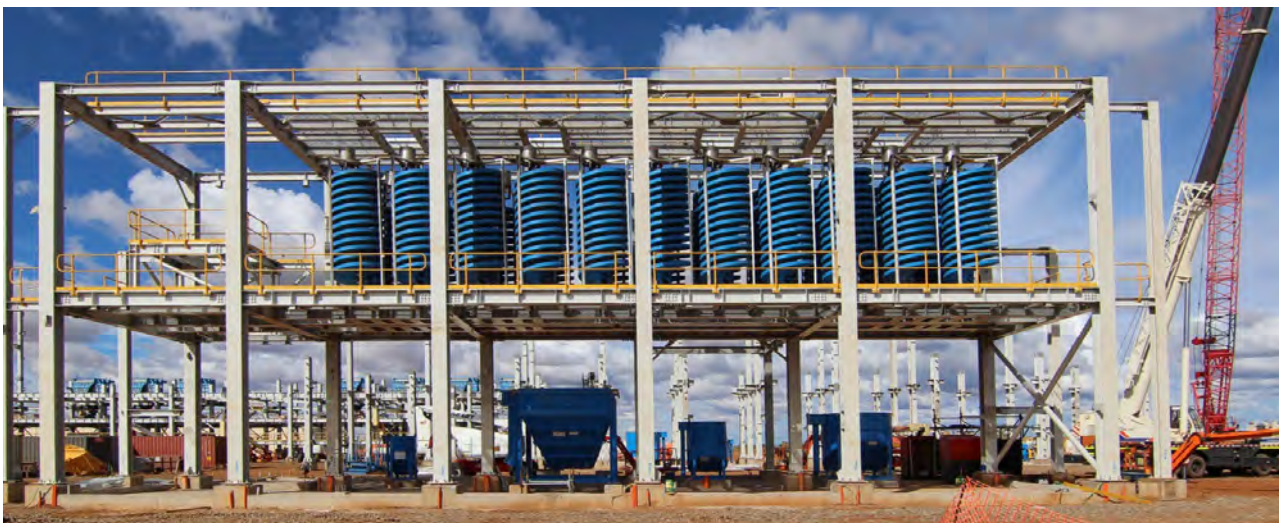
Figure 17: Spirals for removing fine native copper - part of the Gravity Circuit
