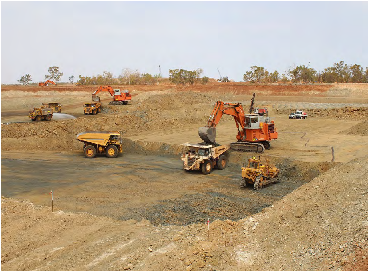
Figure 8: LM1 Pit towards the end of the free-dig period - blast-hole drilling can be seen in the background (right)
