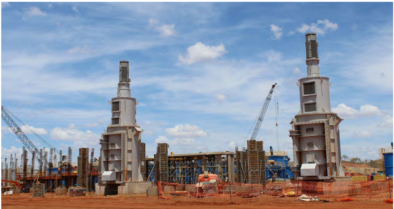
Figure 28: Scrubber Building being erected around the scrubber (top); Gravity Jig Building (middle) and; Vertical Regrind Mills (re-grid circuit for cobalt and magnetite)
