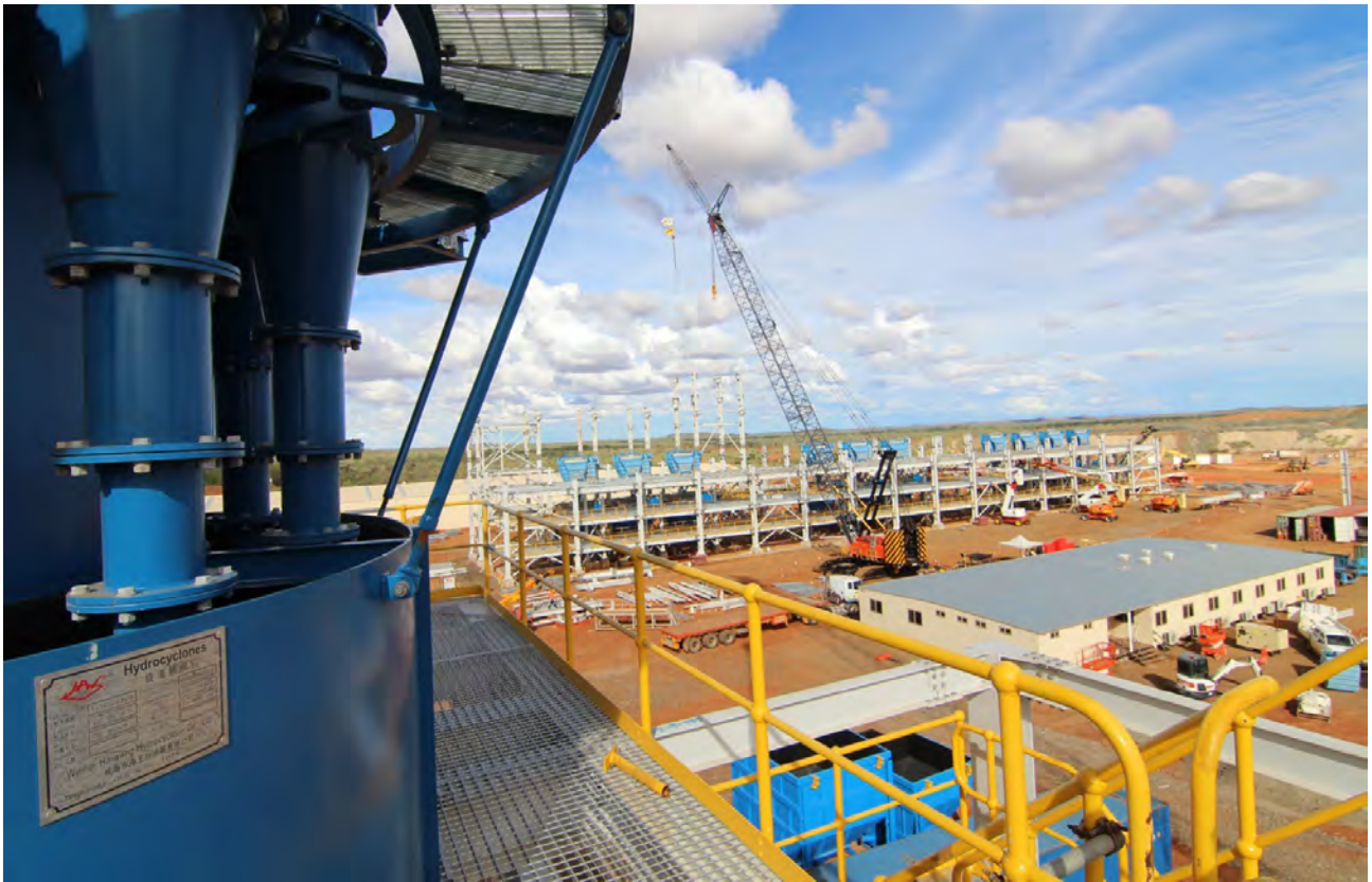
Figure 21: View from the top of the Ball Mill of the Gravity Jig Building in background and Mineral Processing Control Room and Office Complex to the right
