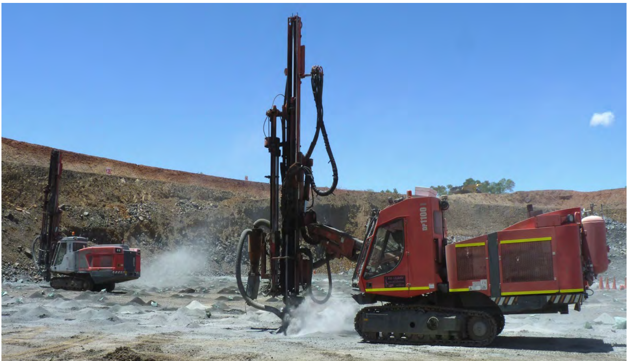
Figure 14: Blast-hole drilling in LM1 - three rigs are currently active in the LM1 pit
