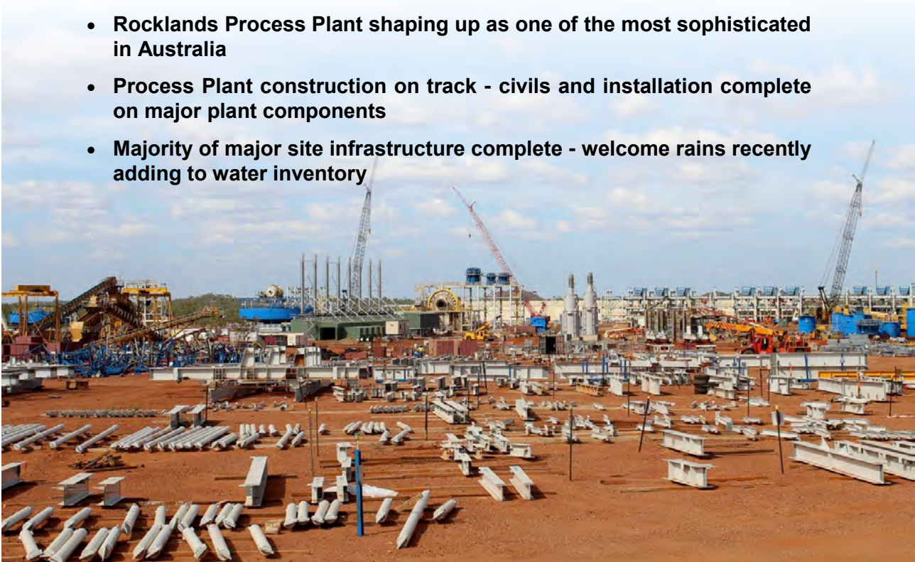
Figure 1: Process Plant growing day-by-day with construction progressing across numerous areas of the Process Plant.
