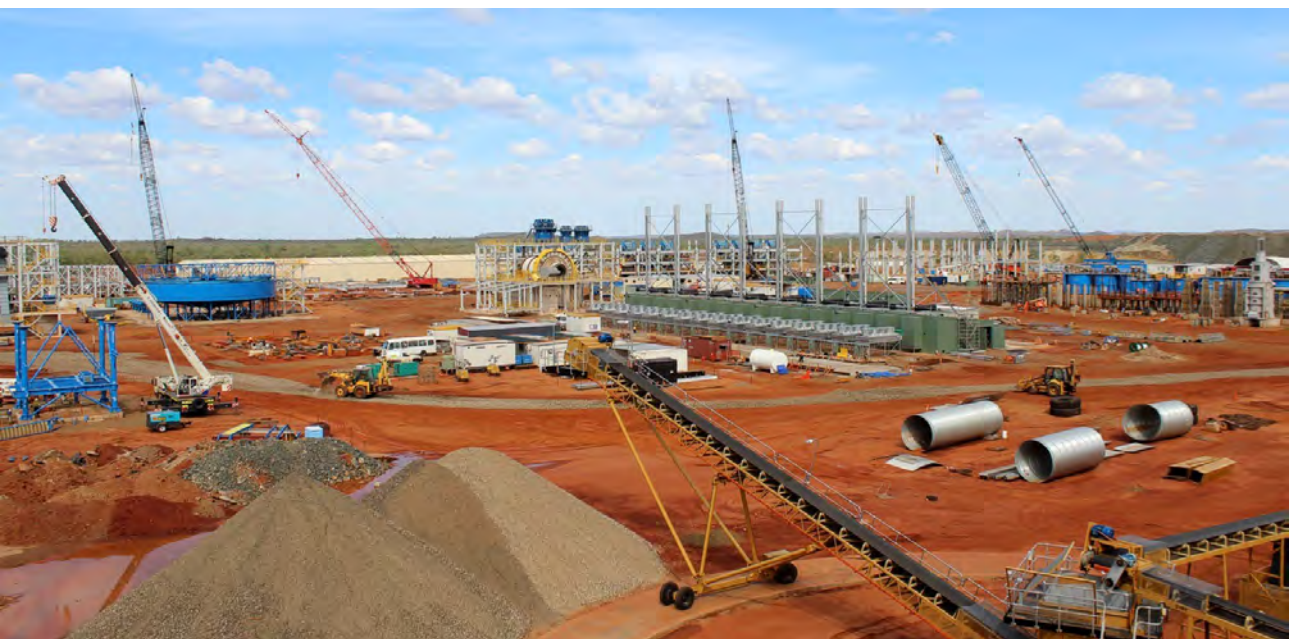
Figure 27: Gravity Jig Building (top image); Thickeners (foreground), Flotation cells (middle distance) and Jig building (far right background) (middle image) and; Crushing Circuit (foreground) Gravity Thickener, Ball Mill, Power Station and Flotation Cells (left to right middle distance).
