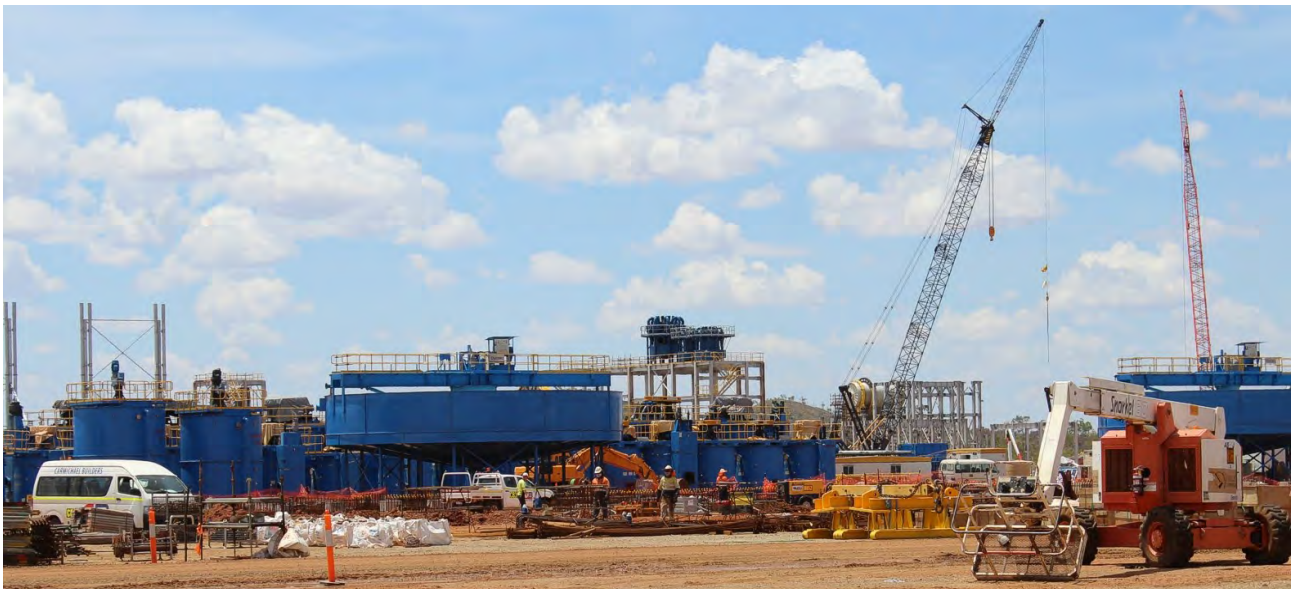
Figure 22 (left to right): Flotation Cells (copper), Concentrate Thickener, Flotation Cells (Pyrite), Ball Mill & Scrubber (background) and another Concentrate Thickener (right)
