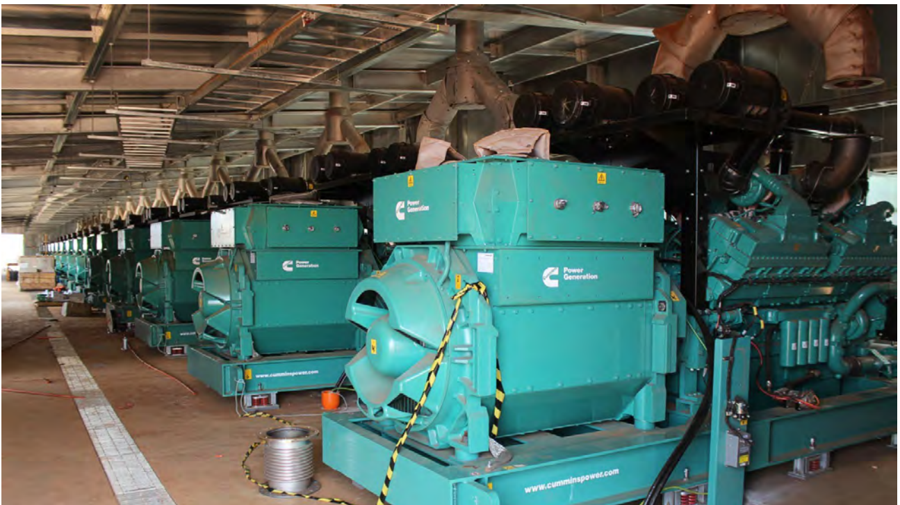
Figure 26: Cummins Power Station - generators installed
