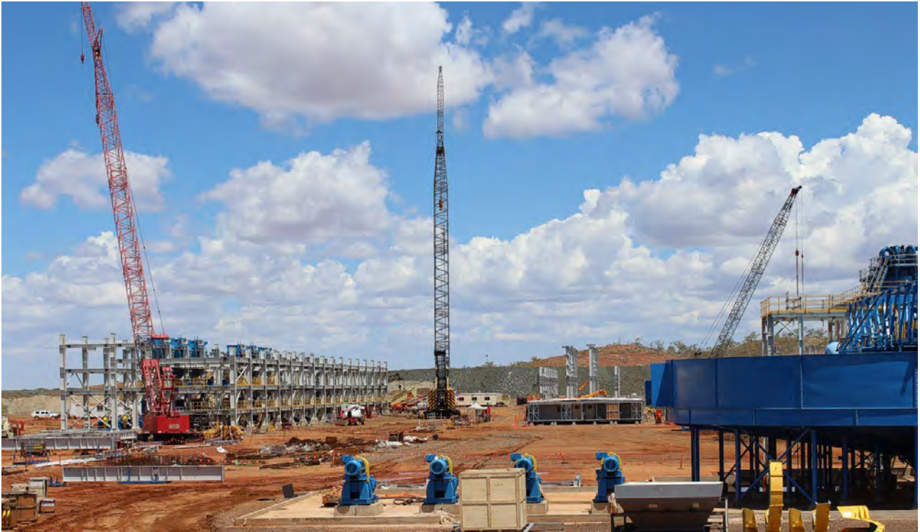
Figure 19: Gravity Jig Building will stand 37m high when completed (left) Mineral Processing Control Room and Office Complex (middle) and Gravity Thickener (right)
