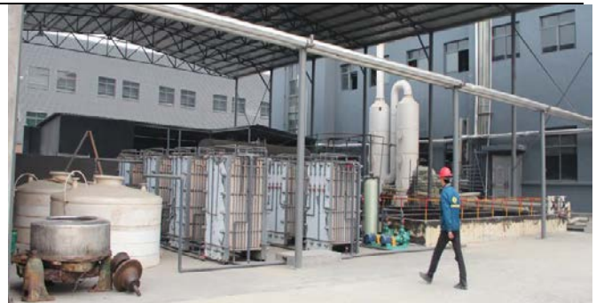
Hengda's chemical recycling facility required for the final flake graphite purification at Yichang.
