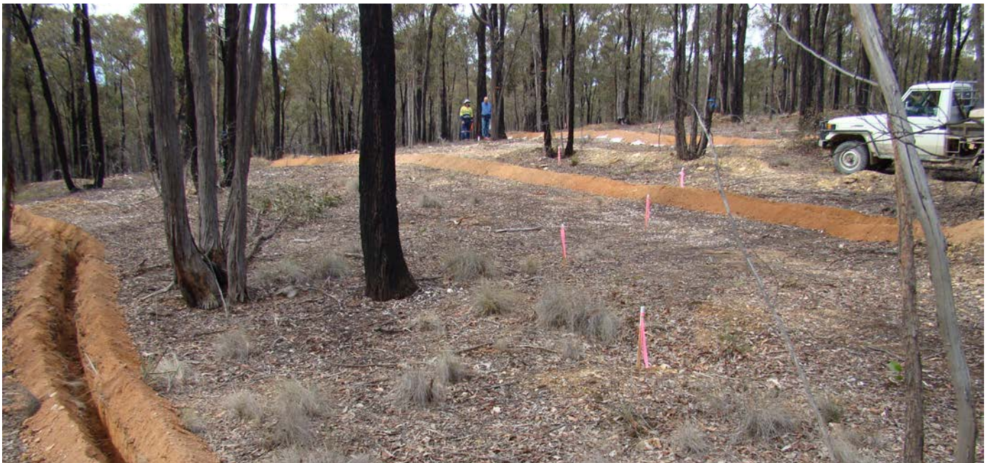
Surface grade control trenching with pit outline at the Pearl Croydon Deposit (April 2014)
