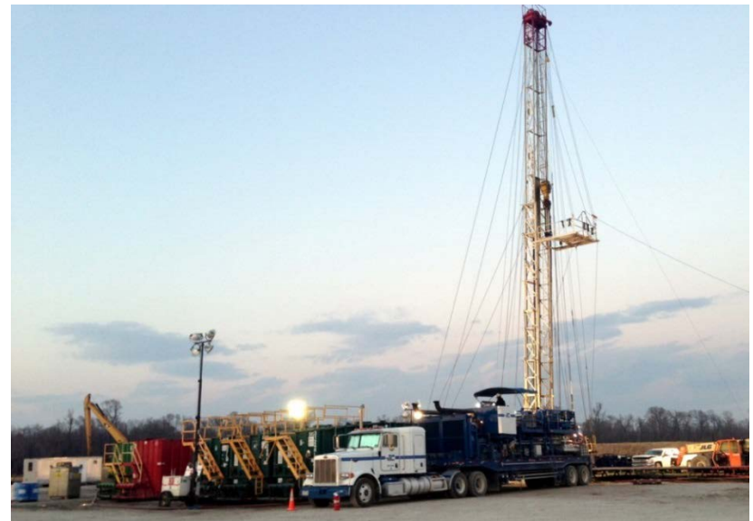
Work over rig running production tubing on the Rosewood Plantation 21H well
