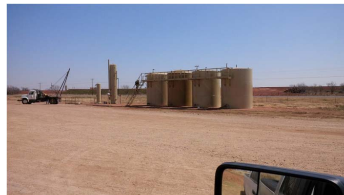
Oil storage facility
