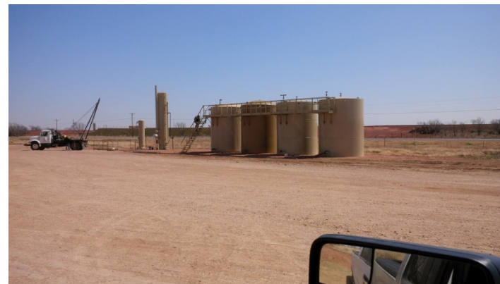
Oil storage facility
